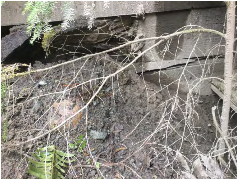
Ballast wall condition at downstream right bank
