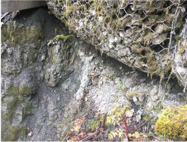
Downstream right bank erosion under gabions
