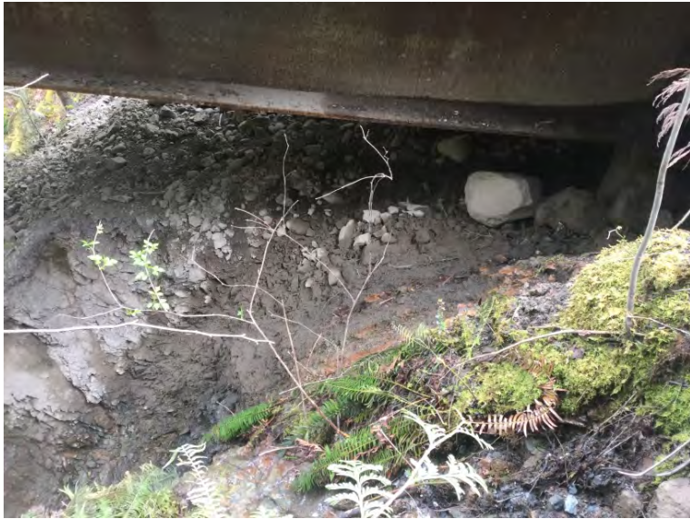
Fill erosion in front of upstream right bank footing
