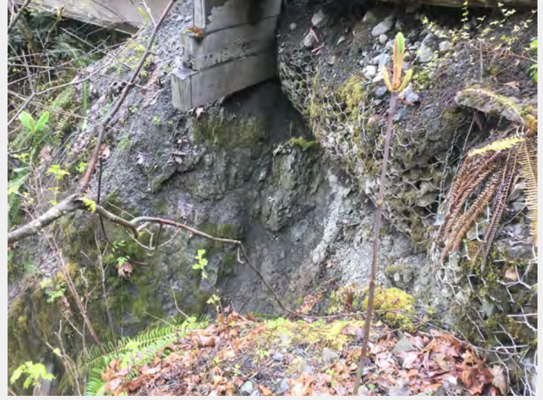
Downstream right bank erosion under gabions
