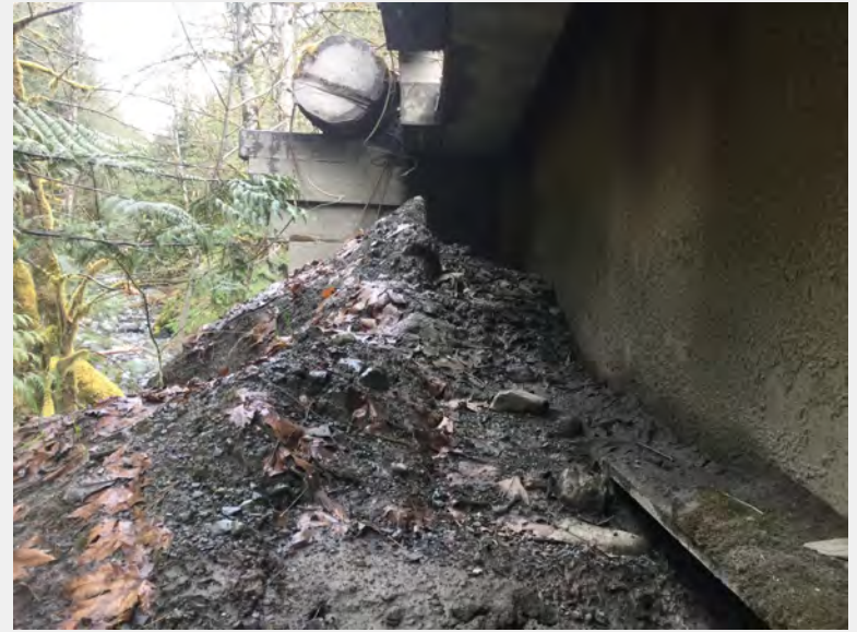
Sediment accumulations on girder bearing at downstream right bank
