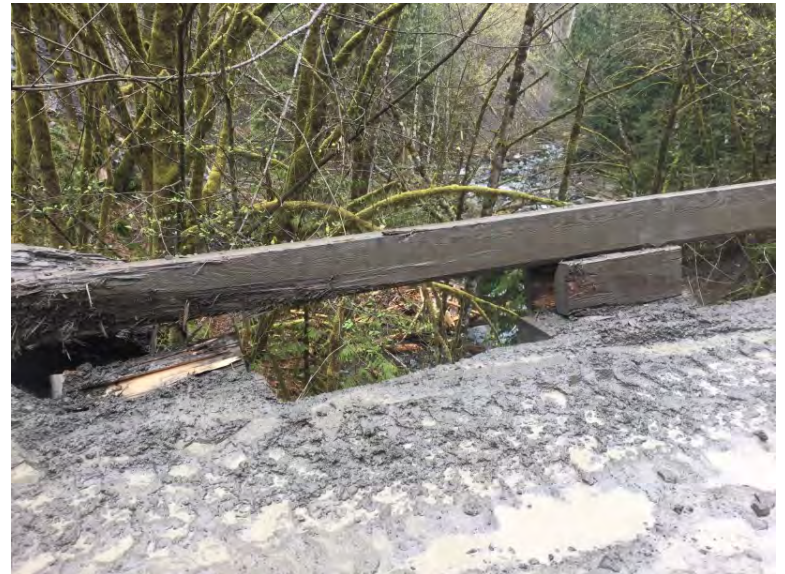
Downstream left bank guardrail damage
