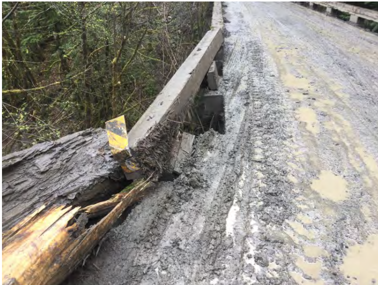
Downstream left bank guardrail damage
